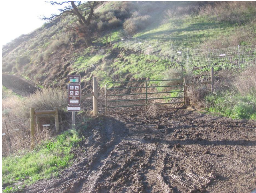
Figure 3. Example of significant rutting and unstable conditions. The indentations were created by a typical emergency response vehicle.
