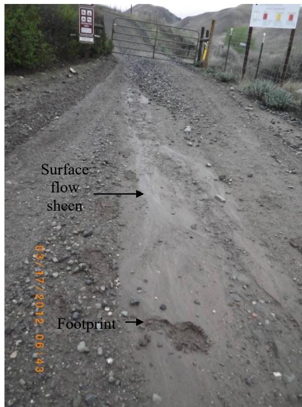
Figure 4. Unstable site conditions. The impression of the footprint and sheen of surface flow suggest the site is not dry enough to reopen.
