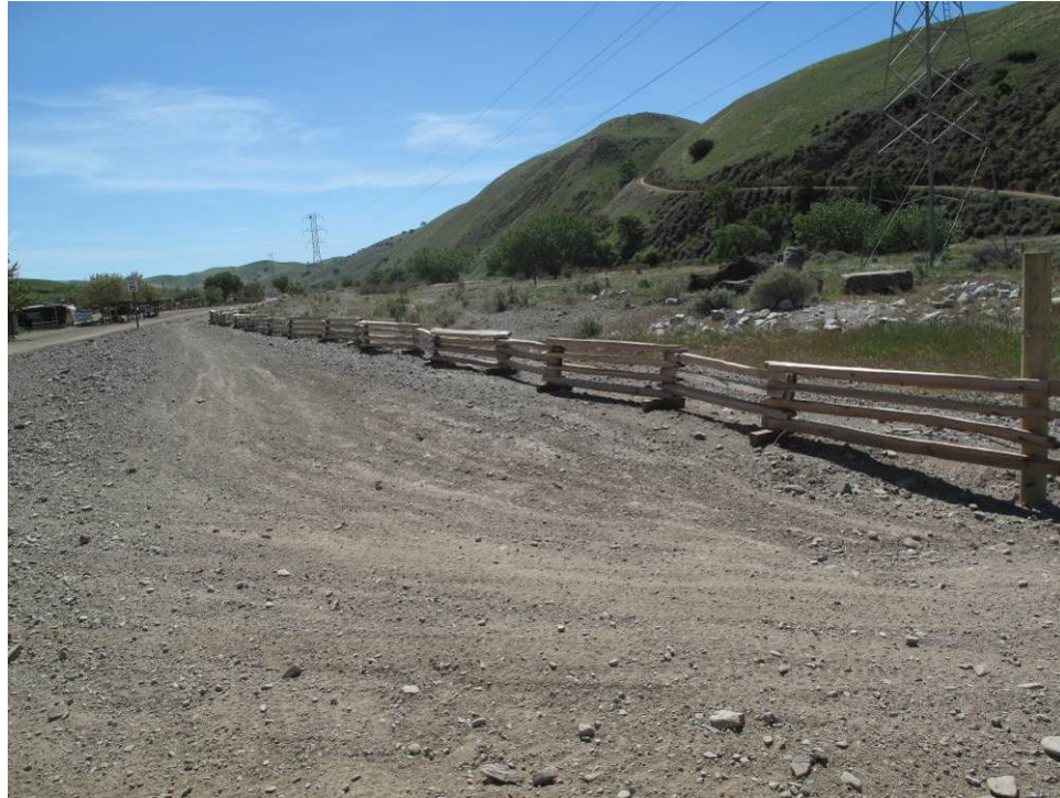
BMP 165-RMA Fence
