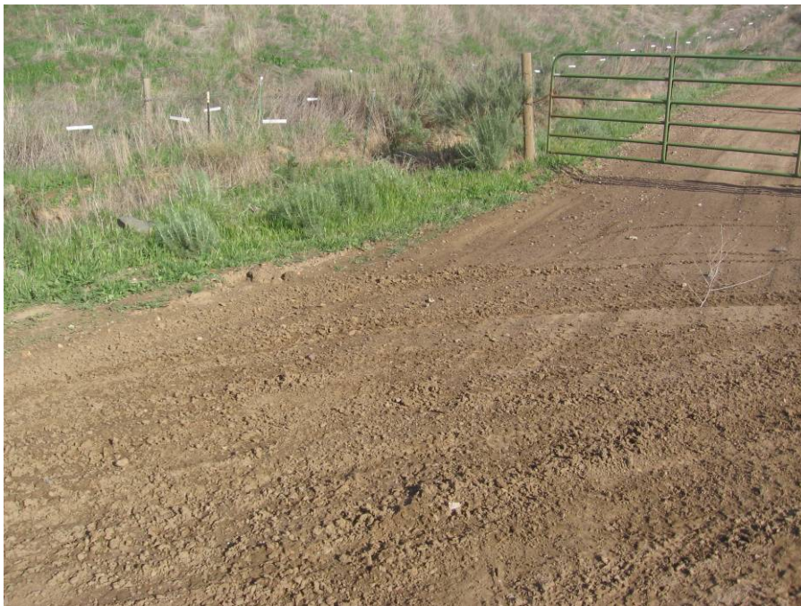
Figure 8: Example of stable conditions. Recent vehicular activity in the foreground show minimal signs of rutting.
