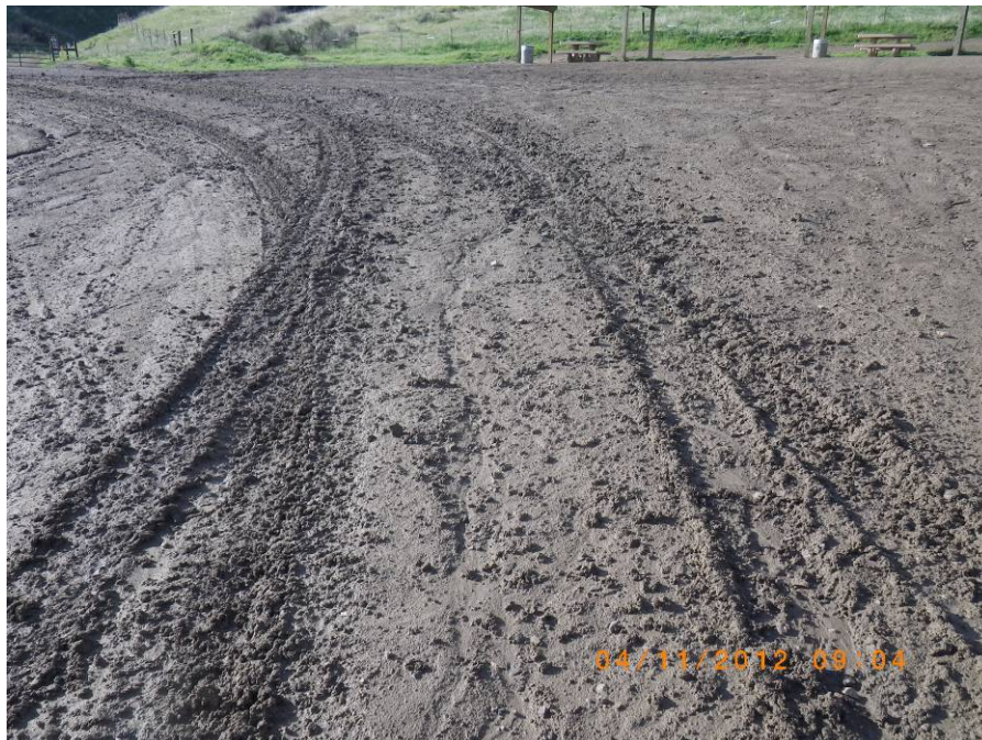
Figure 6. Example of significant rutting and unstable conditions. The indentations were created by a typical emergency response vehicle.
